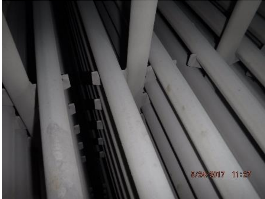
Photo 4 – Boiler bank tubes sitting flat in support lugs on the stringer tubes.
