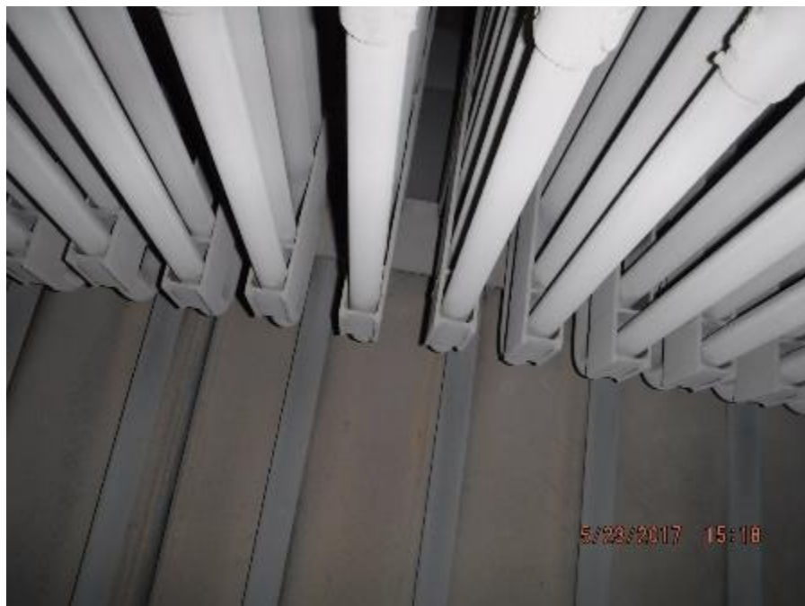
Photo 38 – On front wall of back pass, primary 1 SH element supports are in good condition.
