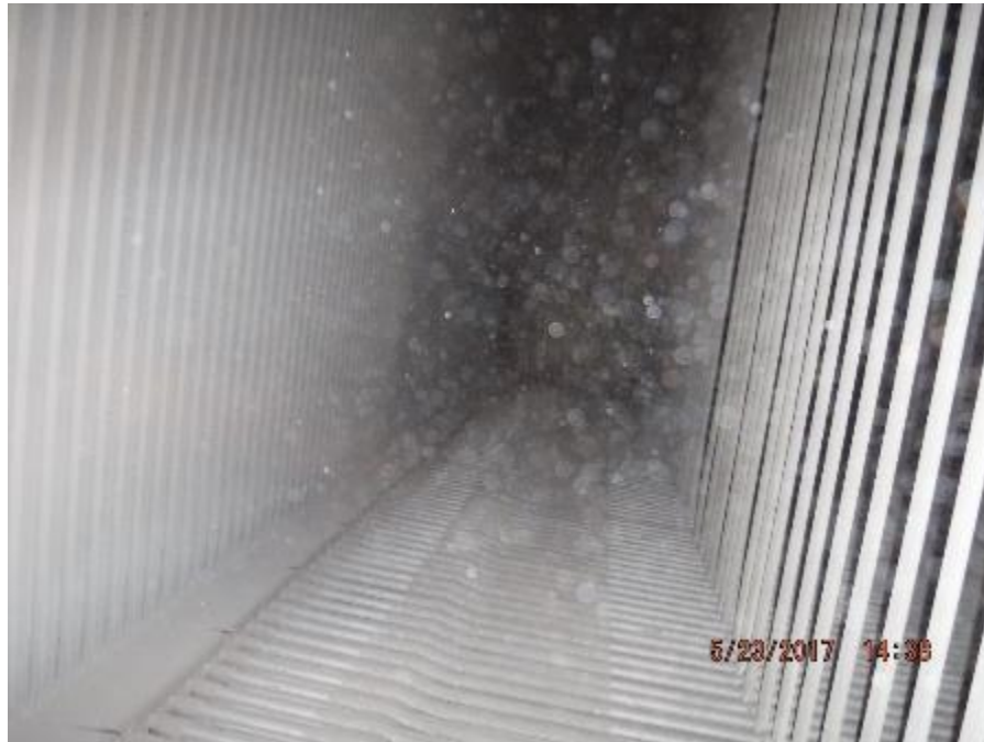
Photo 26 – View of rear wall of back pass superheater enclosure. Tube wall panels are straight. Above P1SH, erosion baffle plates in very good condition.
