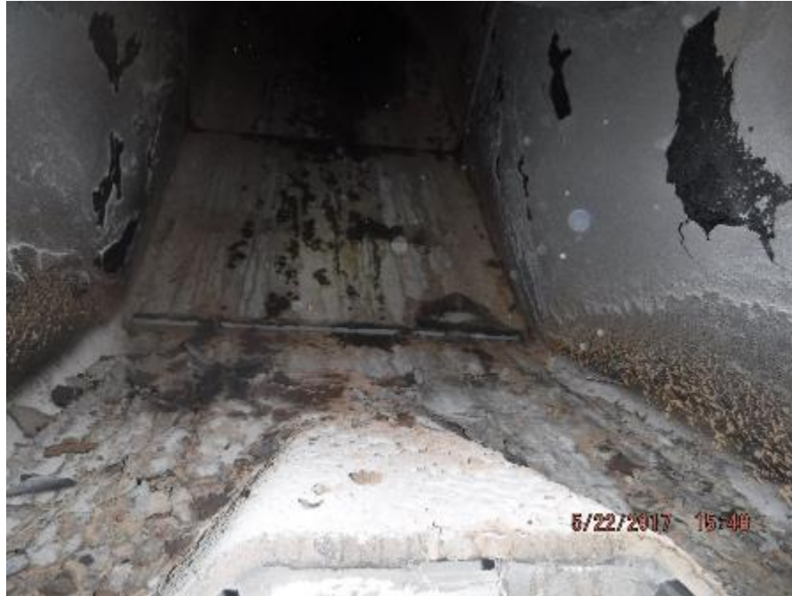
Photo 67 – Depicts very good condition of metal plate work at biomass fuel feed openings.
