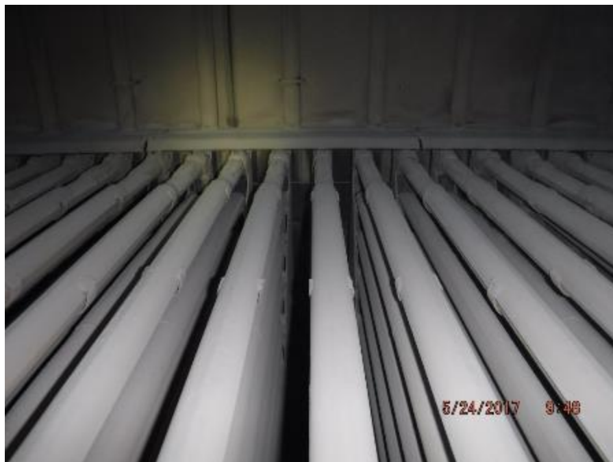
Photo 3 – Top face of boiler bank, elements are straight. No ash deposit build up on tubes or between elements. Tube shields in good condition.
