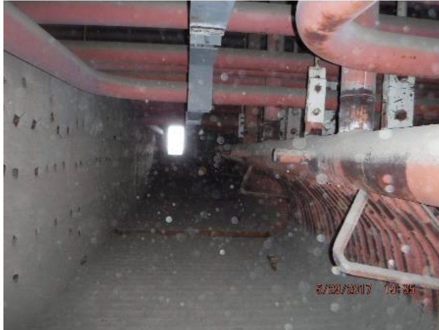
Photo 77 – View across front section of penthouse. Slight dusting of fly ash.
