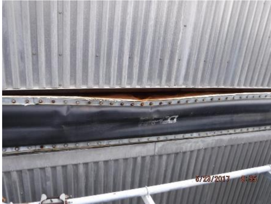
Photo 76 – At flue gas inlet duct to economizer, deformation to the flanges of the expansion joint.
