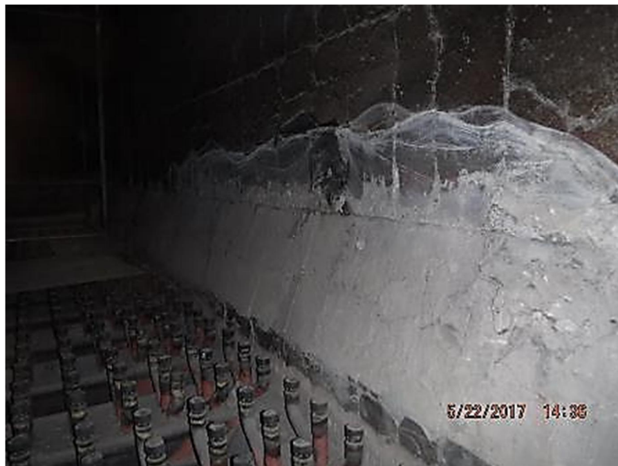
Photos 60 – Lower furnace refractory is in good condition with no repair work required.
