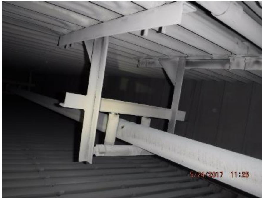
Photo 10 – In boiler bank section, roller guide support for sootblower lance.
