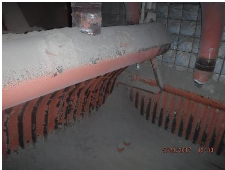
Photo 80 – Front section of penthouse. Fly ash accumulation where roof tubes interface with left side wall tubes.
