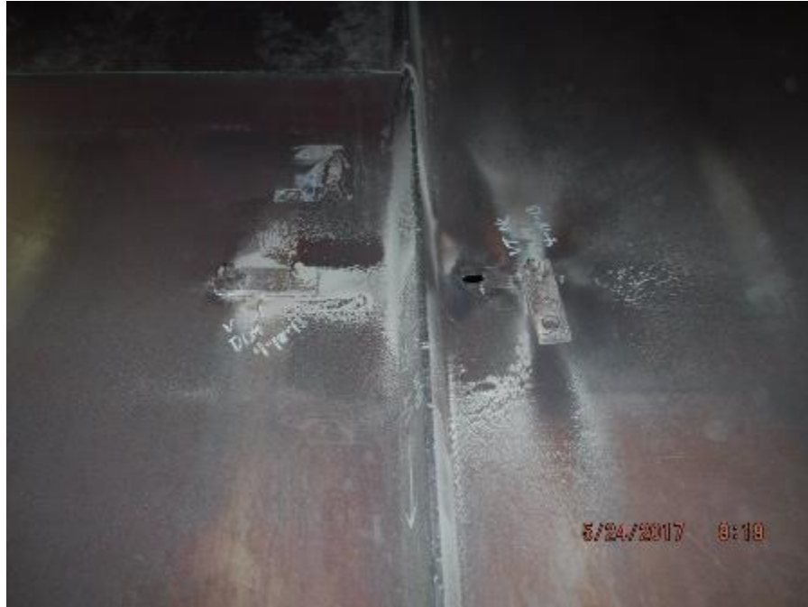
Photo 85 – In nose arch dead air space, broken “U” bolts that is used to secure seal plates to tube in back pass.
