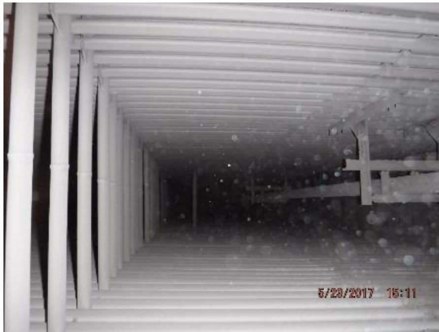
Photo 1 – View is of sootblower lane between P1 superheater and boiler bank. No sagging in boiler bank elements.
