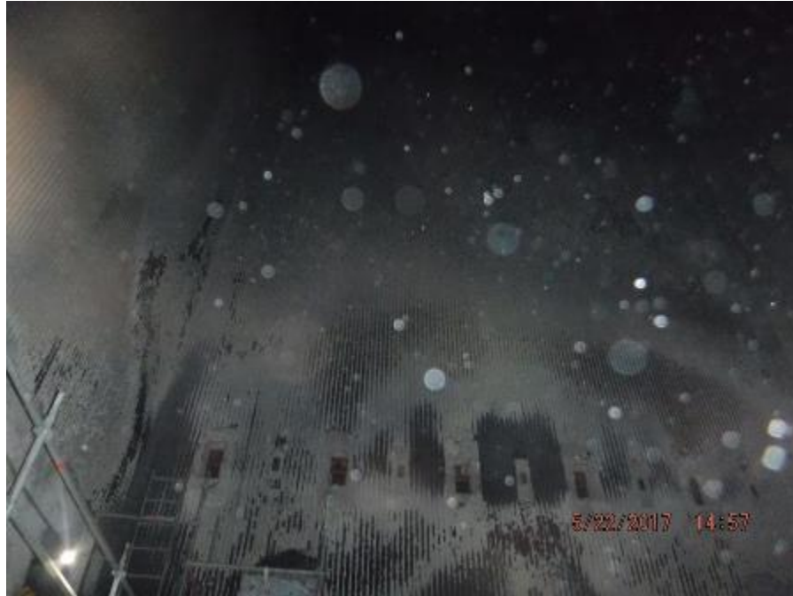
Photo 14 – Lower furnace front wall tube panels are straight with spot areas having slight ash deposits.
