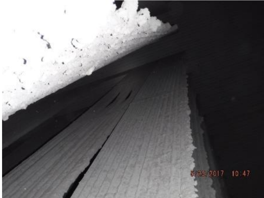
Photo 51 – Secondary superheater element #10; bowed individual tubes in front section of inner tube loop bundle.
