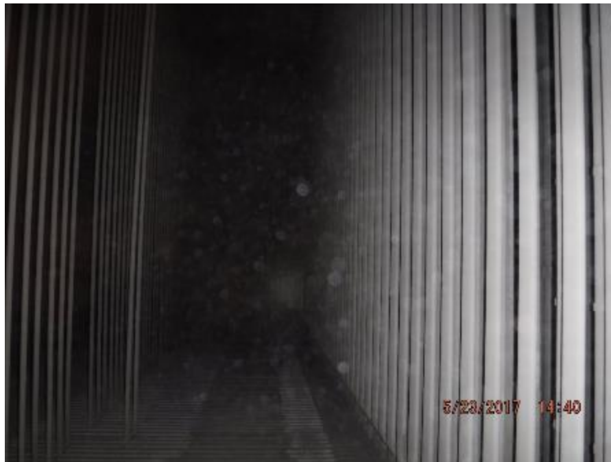
Photo 19 – As viewed from rear side, front to rear alignment of rear wall screen tube rows is good.
