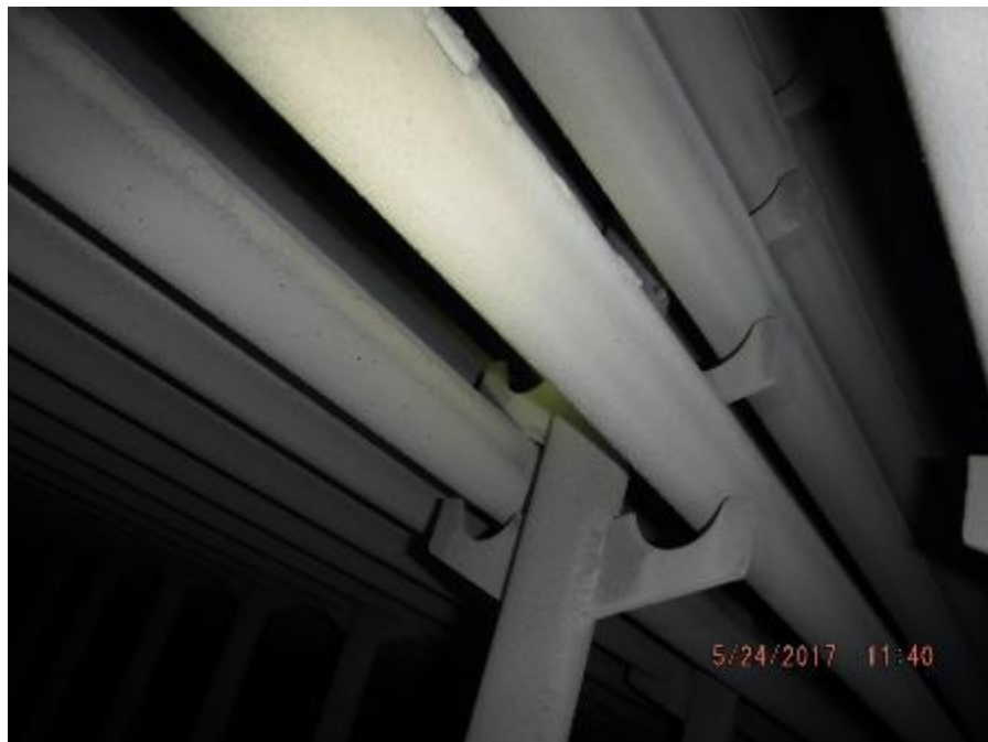
Photo 5 – Boiler bank elements; lower tubes not sitting flat in support lugs on the stringer tubes.
