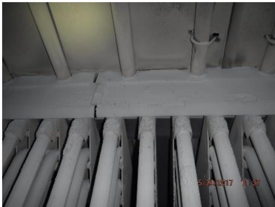
Photo 86 – Front wall of back pass in boiler bank section, broken “U” bolt used to secure nose arch dead air space cavity seal plate to back pass tube.
