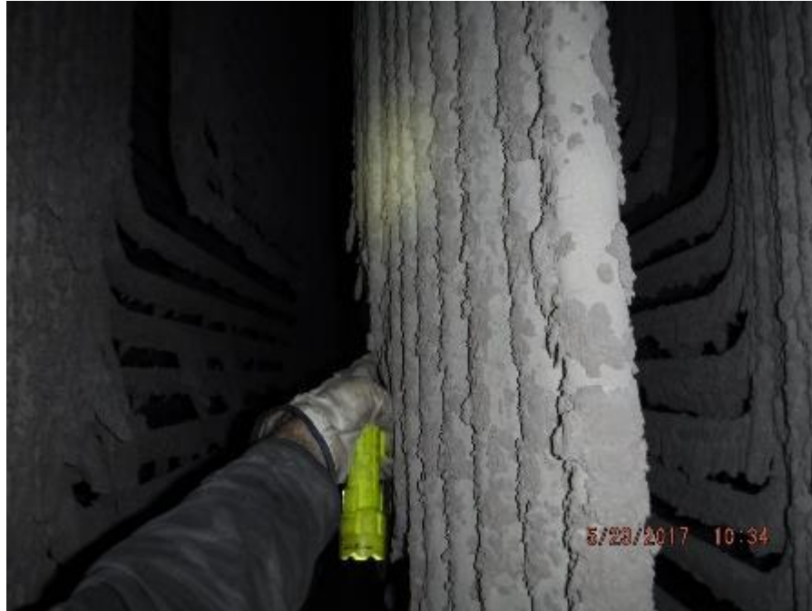
Photo 50 – Secondary superheater element; side direction bowing to lower tube loops in outer tube bundle. View is from rear to front.
