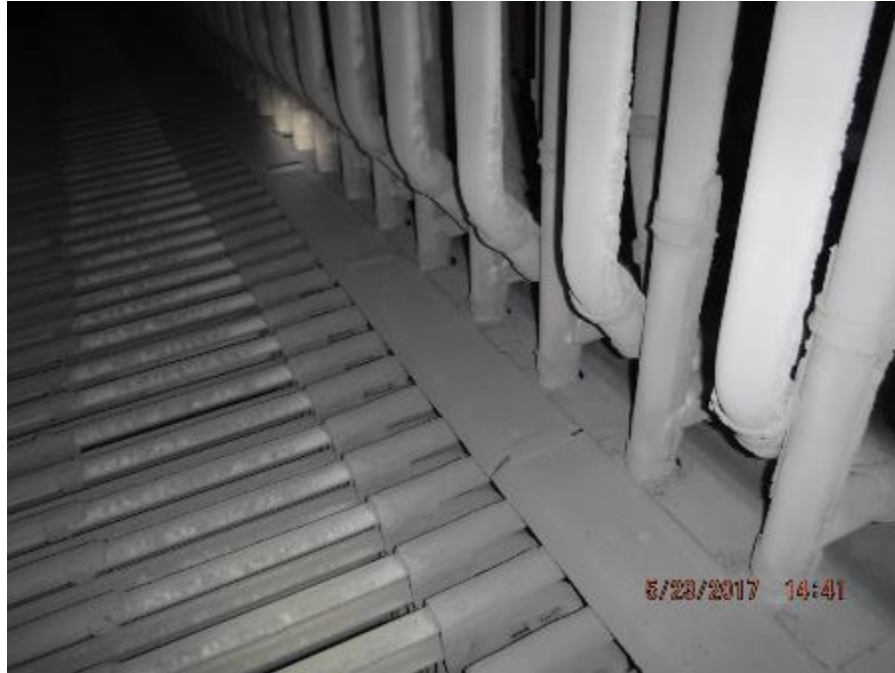
Photo 29 – Directly above P1SH on front wall of back pass superheater enclosure, erosion baffle plates are in very good condition.
