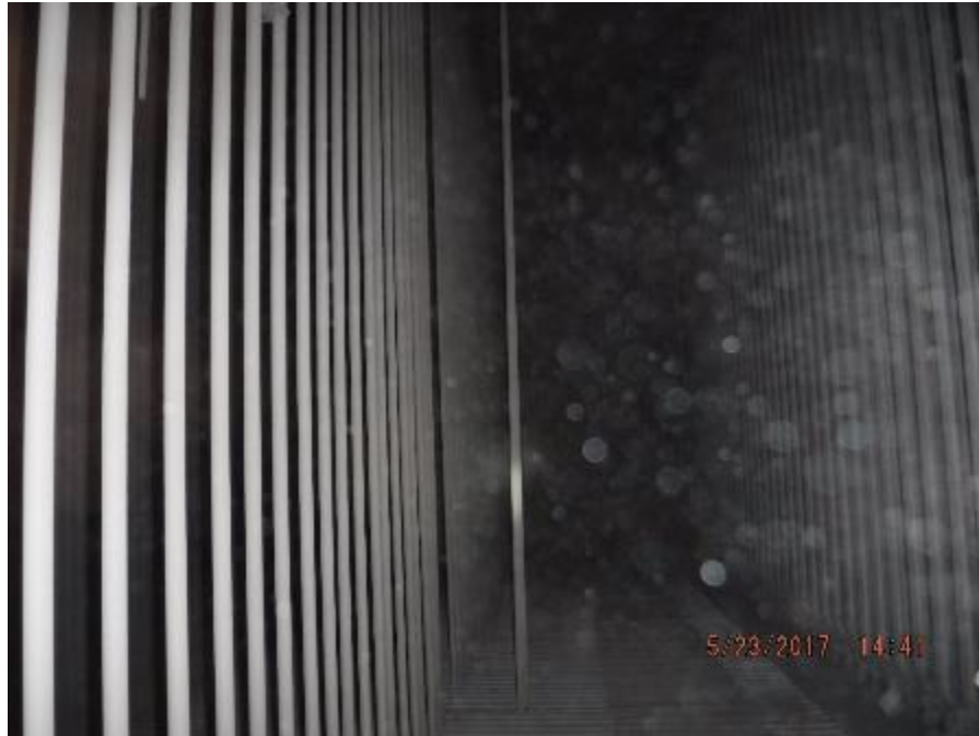
Photo 31 – Front row of SH stringer tubes are straight and in plane.
