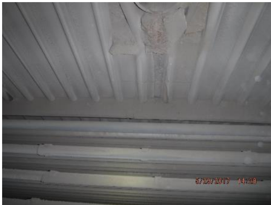
Photo 30 – Directly above P1SH on left wall of back pass superheater enclosure, erosion baffle plates are in very good condition.
