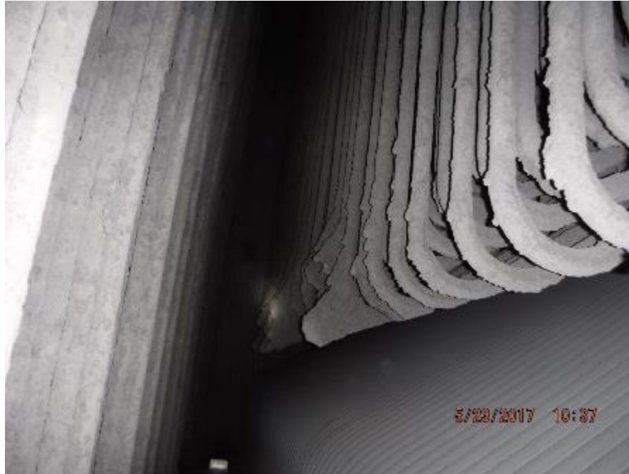
Photo 53 – Front to rear alignment of finishing SH elements is good. View is right to left with finishing superheater on right side of photo.
