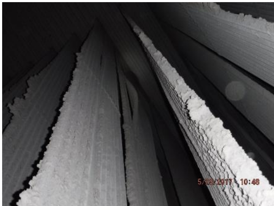
Photo 52 – Secondary superheater element #23; bowed individual tube in front section of inner tube loop bundle.
