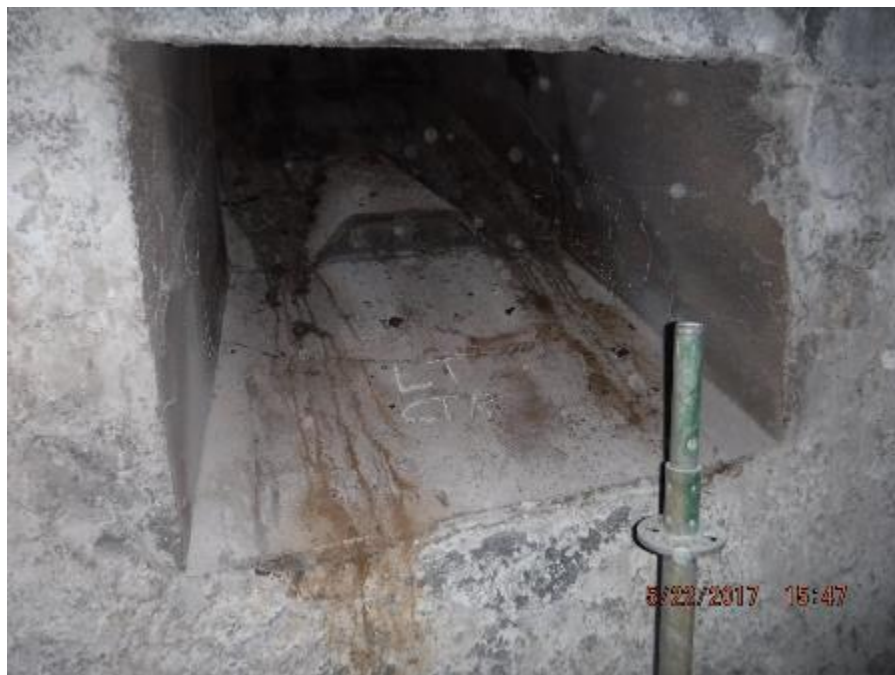
Photo 66 – Depicts very good condition of metal plate work at biomass fuel feed openings.
