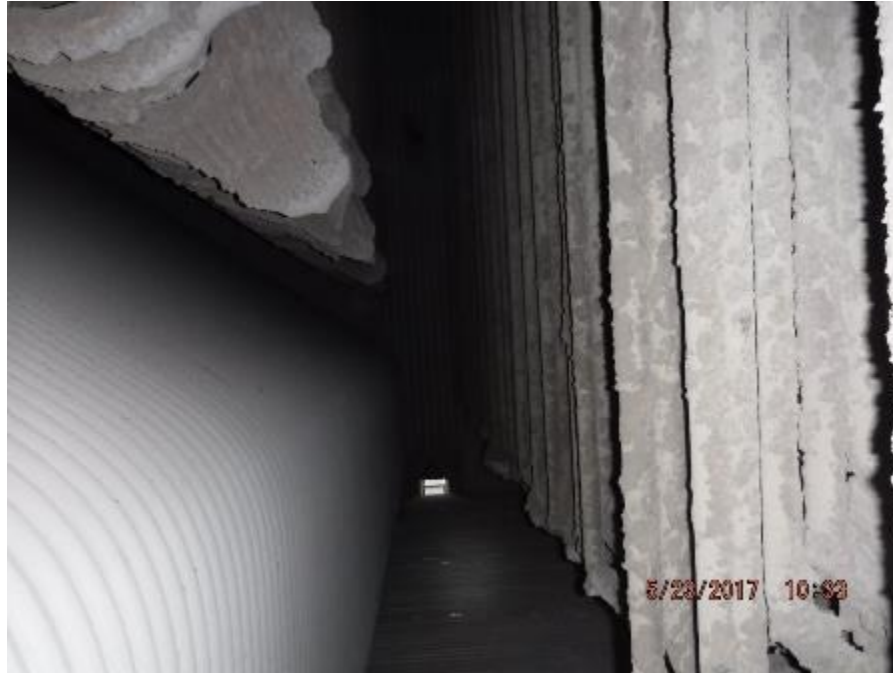
Photo 44 – Looking across rear side of secondary superheater, elements are all in line.
