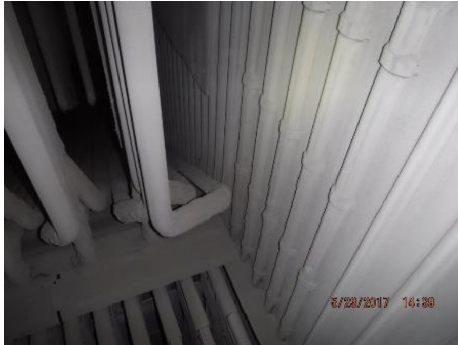
Photo 28 – Tube shields are in good condition on back pass superheater enclosure side wall tubes near rear wall screen.
