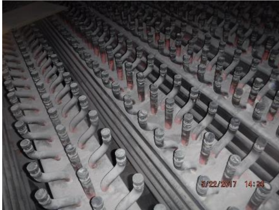
Photo 13 – View of Hybex beam floor tubes.
