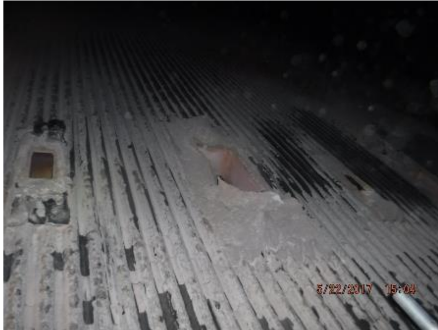
Photo 70 – Secondary air nozzles show no signs of heat warping. Some ash agglomeration built up around opening.
