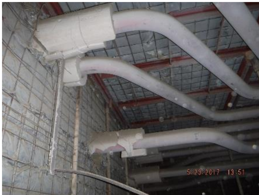
Photo 83 – In rear section of penthouse, sections of calsil insulation block broken off boiler bank riser pipes.
