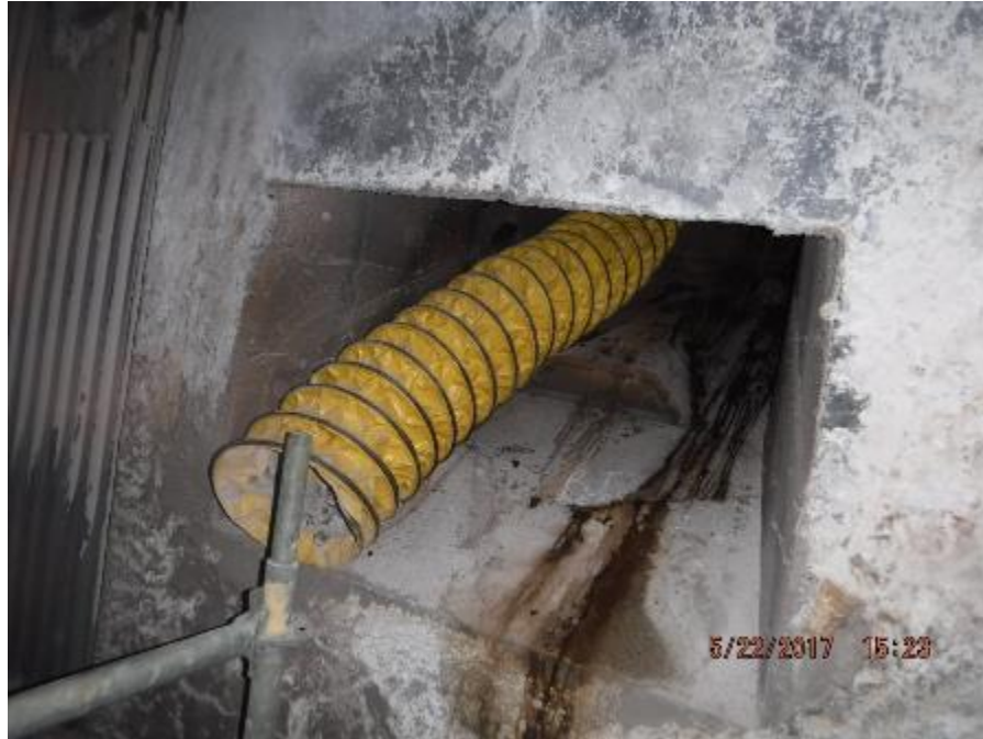
Photo 65 – Depicts general condition of refractory at biomass fuel feed openings. Refractory is in very good condition at all feed openings.
