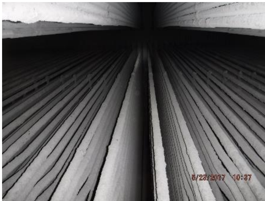
Photo 54 – Side to side alignment between the finishing SH elements is good. Handcuff clamps are in good condition.
