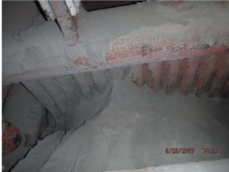
Photo 79 – Front section of penthouse. Next to right side wall, fly ash accumulation in space between roof header and front wall header.
