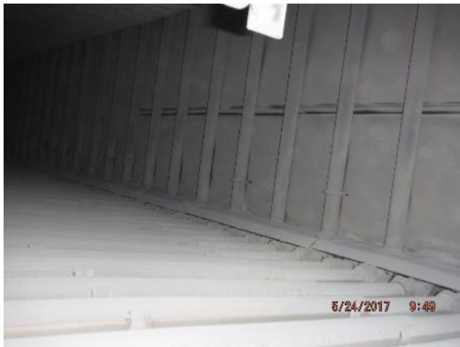
Photo 9 – On top face of boiler bank, front wall erosion baffles in very good condition.
