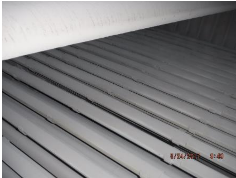
Photo 8– On top face of boiler bank below sootblower lance, tube shields are in good condition, firmly attached and correctly positioned.
