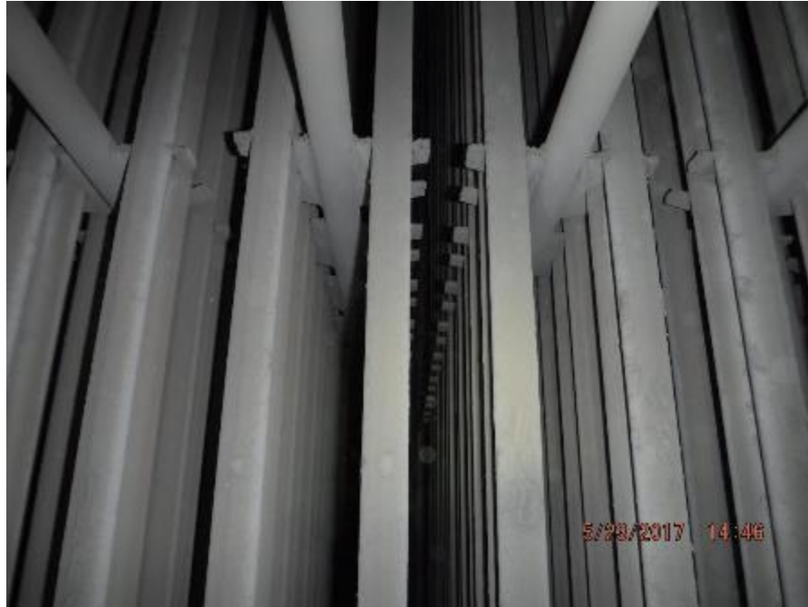
Photo 37 – Primary 1 SH tubes are sitting flat in their support lugs off the stringer tubes.
