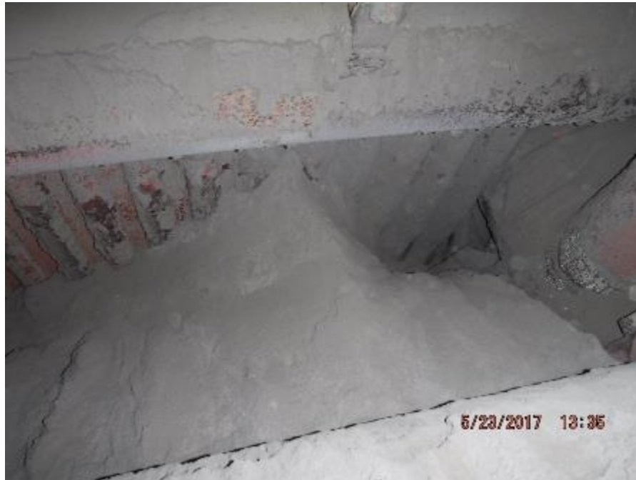
Photo 81 – Front section of penthouse. Next to left side wall, fly ash accumulation in space between roof header and front wall header.
