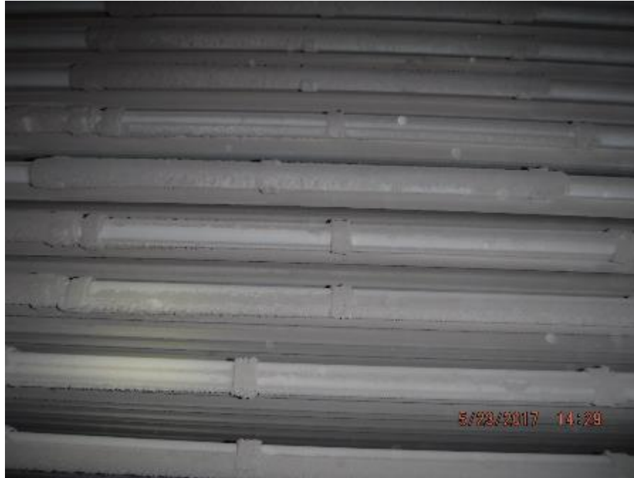
Photo 40 – Primary 1 SH element top tubes, some tube shields rolled out of position.
