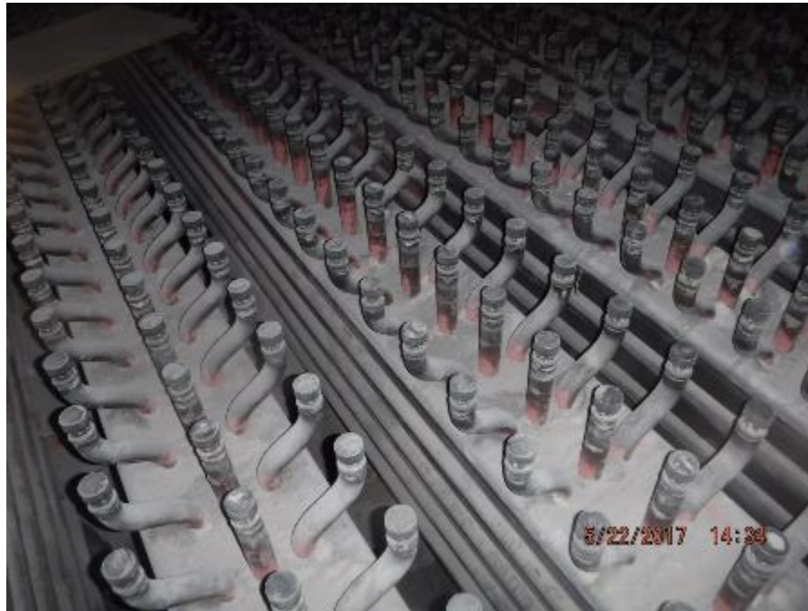
Photo 57 – View of lower furnace tuyeres. The tuyeres are in very good condition.
