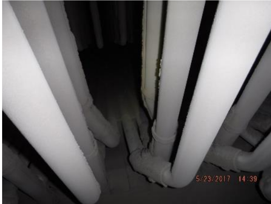
Photo 22 – On screen tubes, tube shields show no heat degradation or erosion thinning and are firmly attached.
