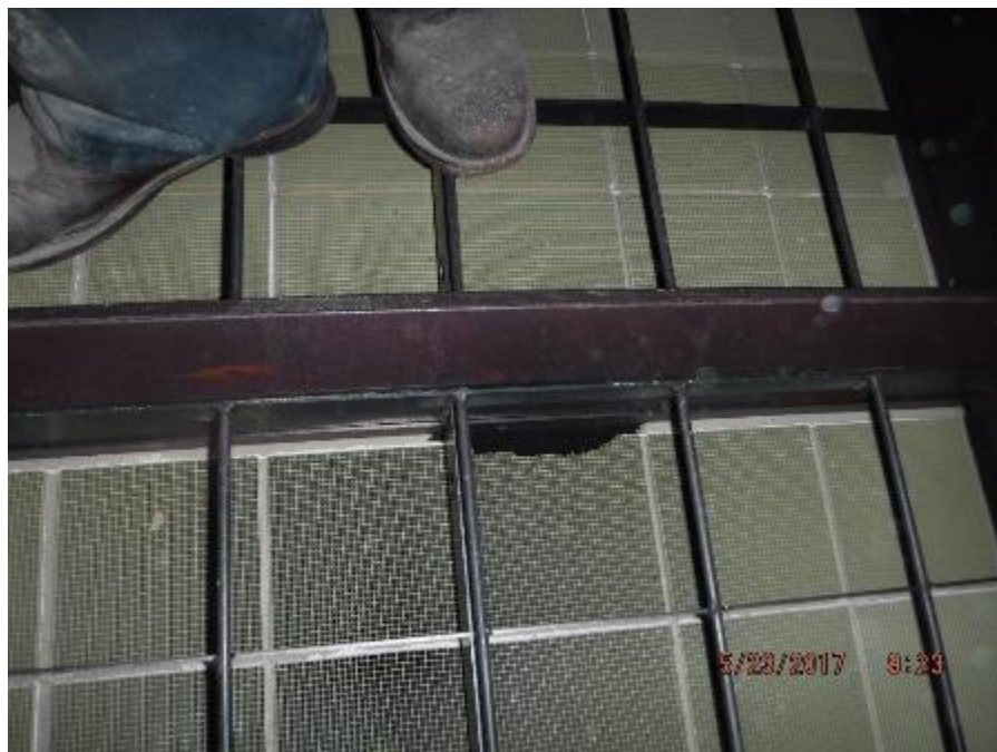
Photo 74 – Small section broke off catalyst basket.
