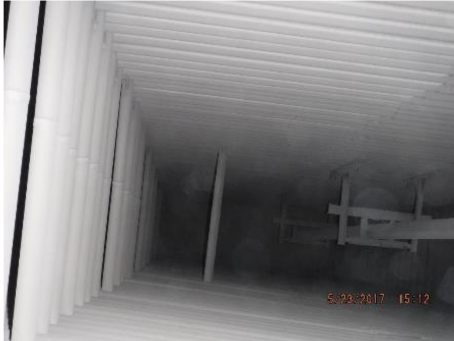
Photo 35 – View across bottom face of primary 1 SH. No downward sag in elements.
