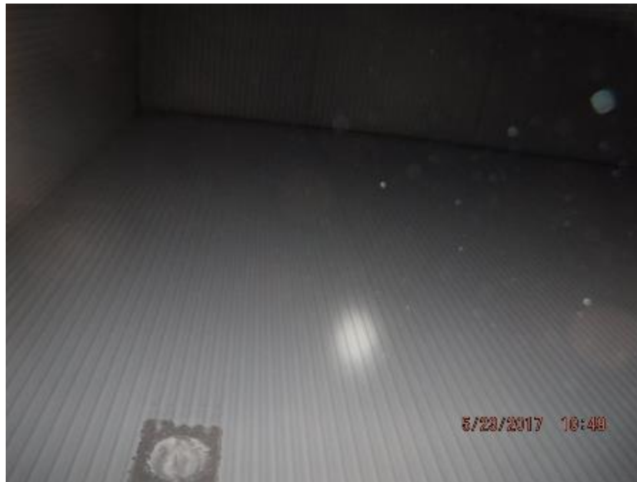
Photo 16 – Upper furnace waterwall tube panels are straight.
