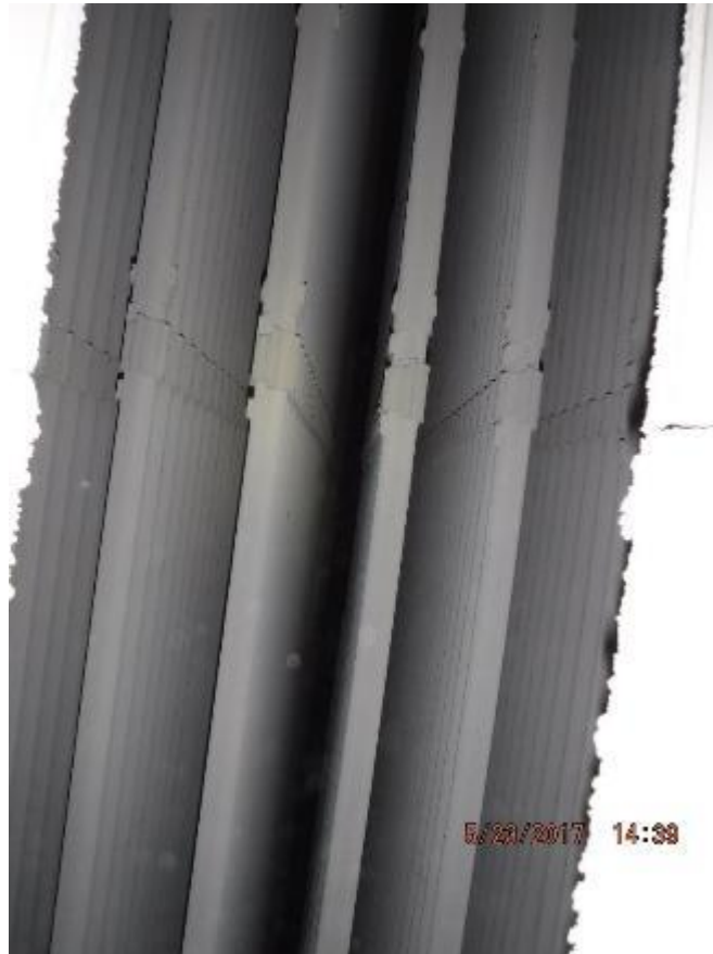
Photo 43 – As viewed looking through the back pass rear wall screen tubes, primary 2 SH element hand cuff clamps are in good condition.
