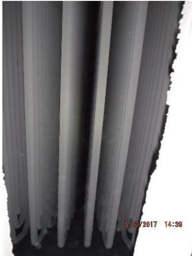
Photo 42 – As viewed looking through the back pass rear wall screen tubes, primary 2 SH element spacing is good. Tube shields are in good condition.
