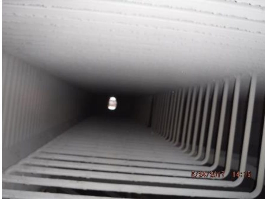
Photo 2 – View of lower face of boiler bank. No sagging in boiler bank elements.
