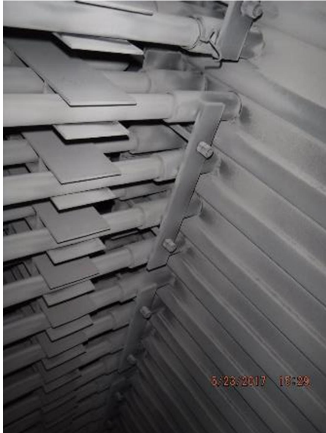
Photo 39 – On rear wall of back pass, primary 1 SH element supports are in good condition.
