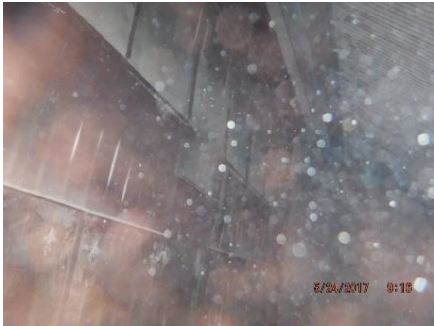
Photo 84 – View of nose arch dead air space. The seal plates are in good condition with no appreciable heat warping.
