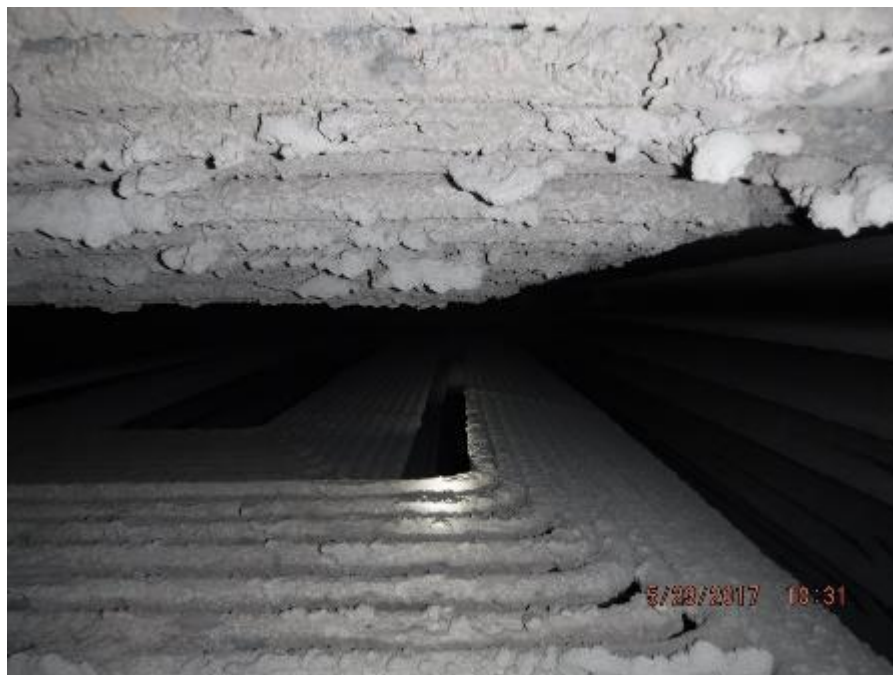
Photo 49 – Secondary superheater element; side direction bowing to lower tube loops in outer tube bundle. View is looking up.
