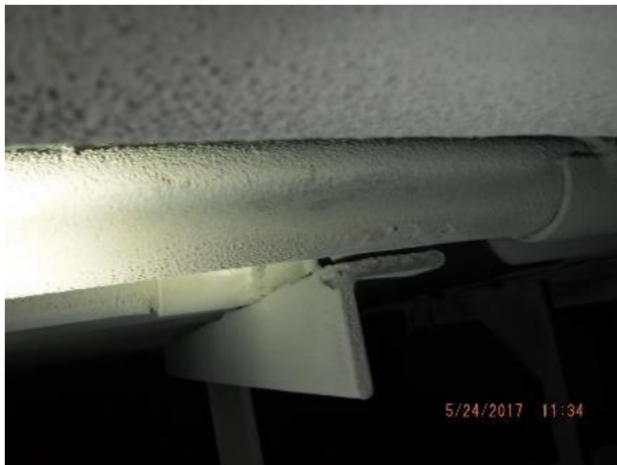
Photo 12 – Roller guide support for sootblower lance; end of mounting angle iron extends over to below tube. Slight gap there. No tube shield there.
