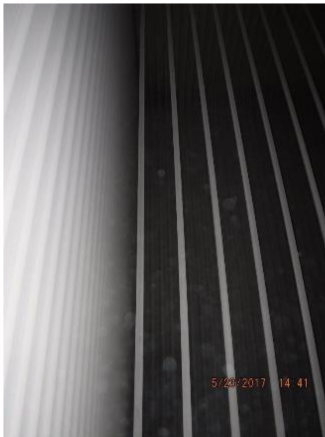
Photo 25 – View of left side wall of back pass superheater enclosure. Tube wall panels are straight.
