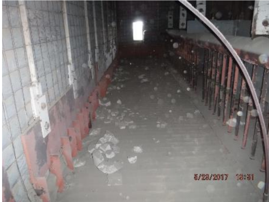
Photo 82 – Slight amount of fly ash accumulation in rear section of penthouse.
