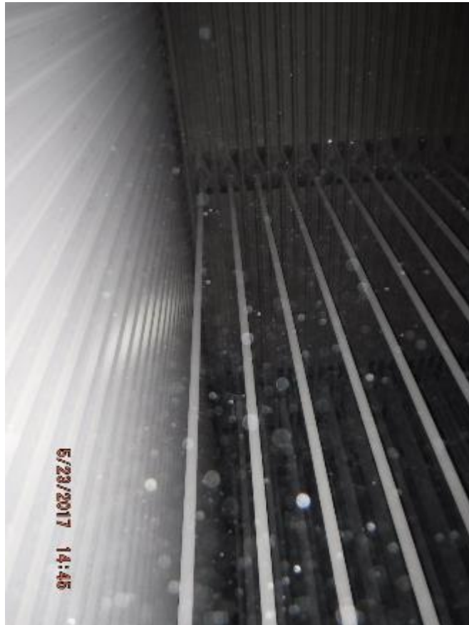
Photo 27 – View of right side wall of back pass superheater enclosure. Tube wall panels are straight.
