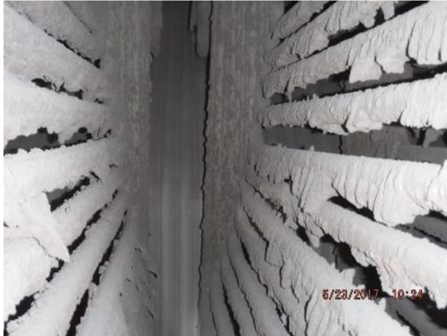
Photo 46 – Secondary superheater element; side direction bowing to lower tube loops in outer tube bundle. View is from front to rear.
