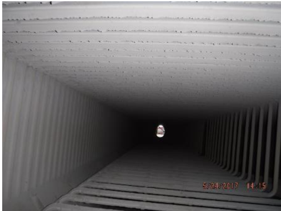
Photo 33 – On horizontal run of SH stringer tubes, tubes are straight and tube shields are in good condition.
