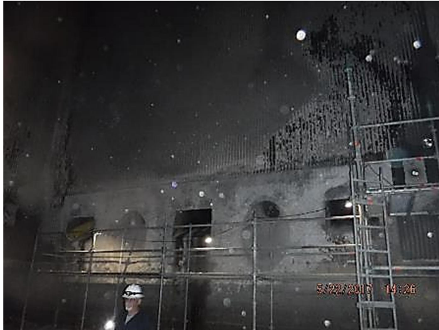
Photo 61 – Lower furnace refractory is in good condition with no repair work required.
