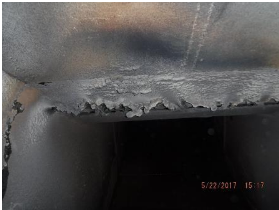
Photo 68 – Biomass fuel feed openings; hardened ash deposits partially blocking off upper sweep air opening slot.
