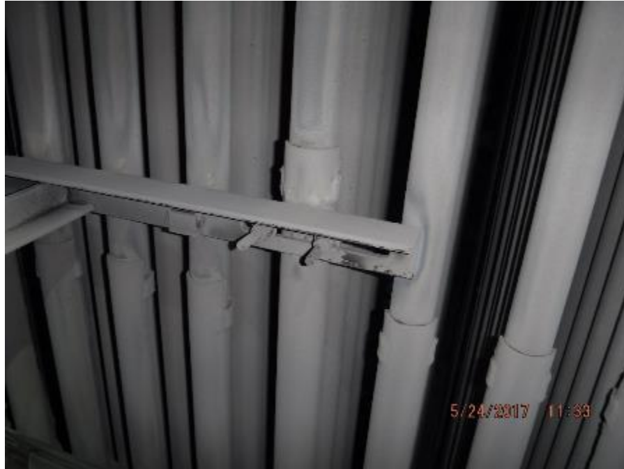
Photo 11 – In boiler bank section; roller guide support for sootblower lance is attached to tubes by “U” bolts.
