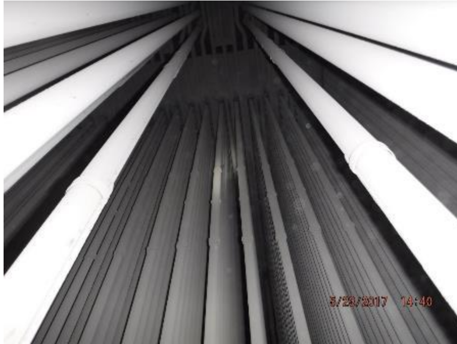
Photo 41 – As viewed looking through the back pass rear wall screen tubes, primary 2 SH element spacing is good. Tube shields are in good condition.
