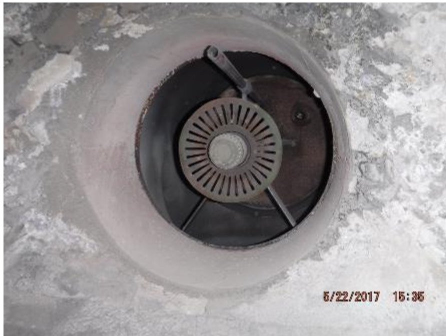
Photo 69 – View of start-up burner opening. Burner throat refractory and diffuser are in good condition.
