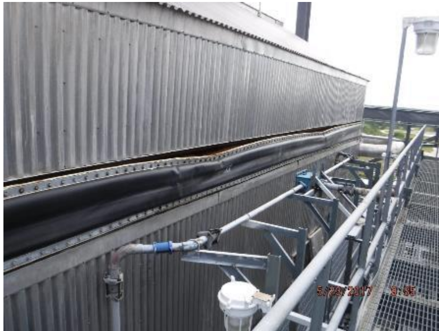
Photo 75 – At flue gas inlet duct to economizer, deformation to the flanges of the expansion joint.
