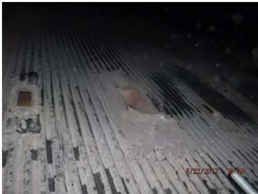
Photo 15 – Lower furnace front wall tube panels are straight with spot areas having slight ash deposits.
