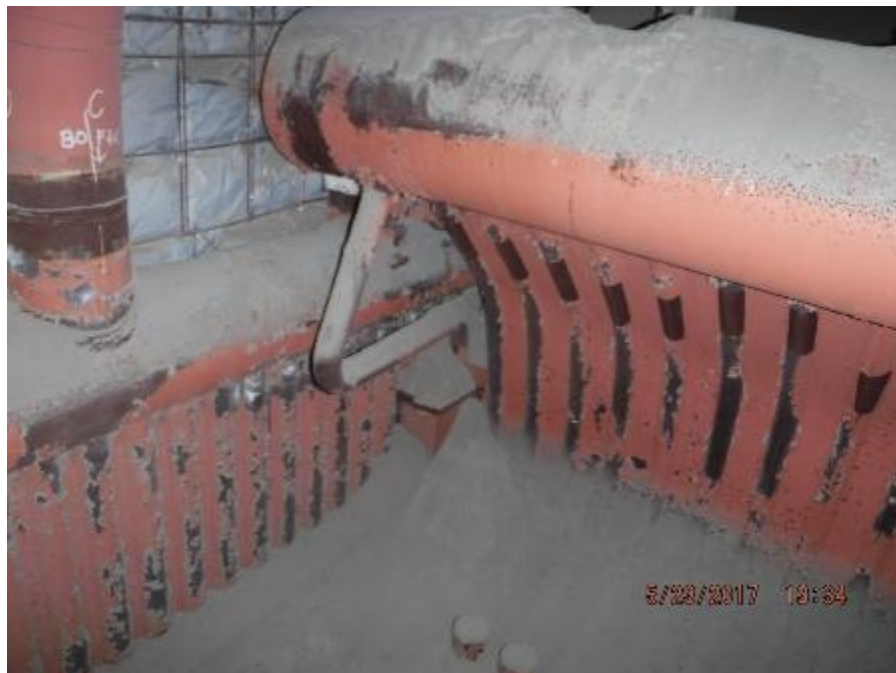
Photo 78 – Front section of penthouse. Fly ash accumulation where roof tubes interface with right side wall tubes.
